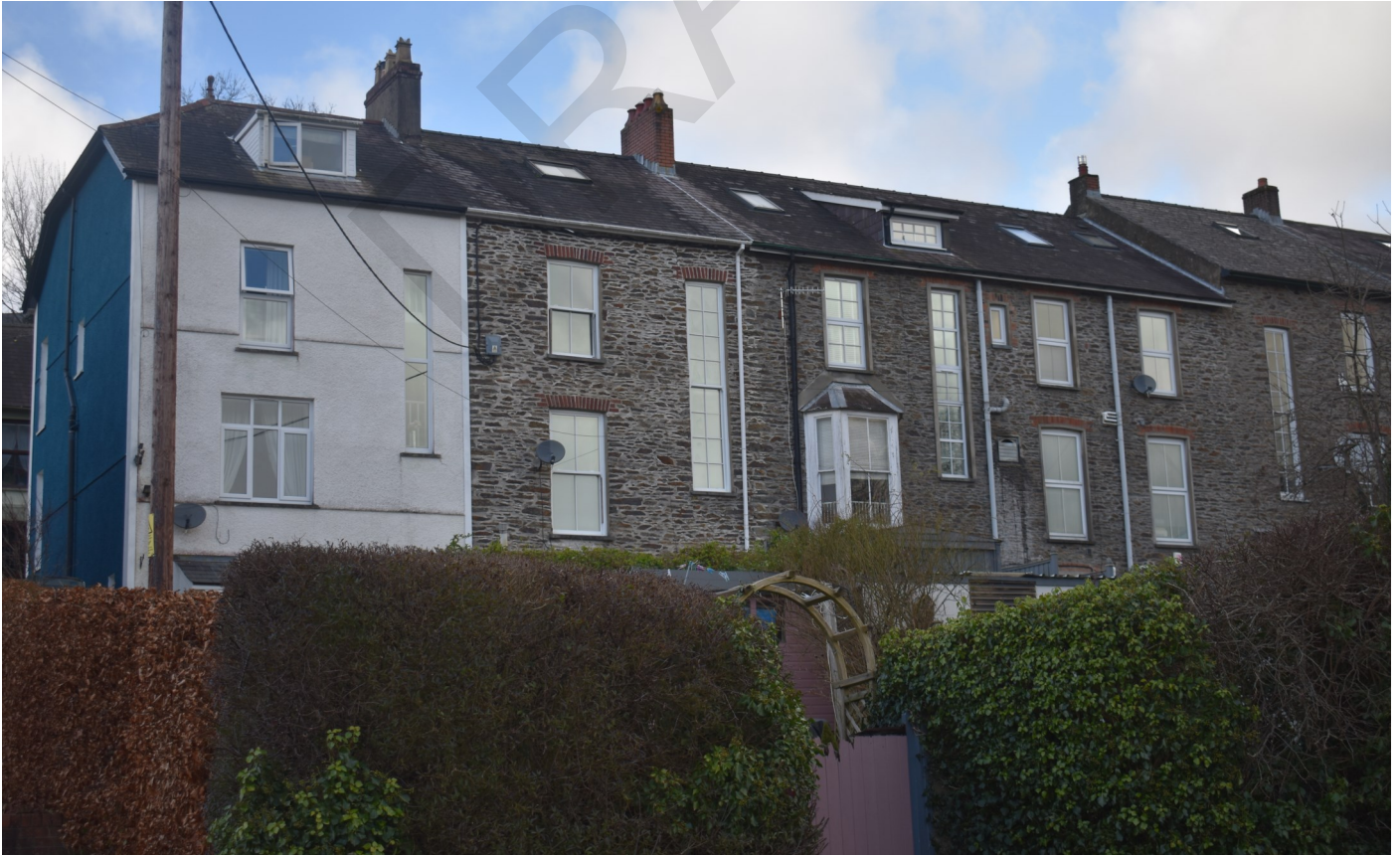
Fig. 7 The rear elevations of properties which front onto King Street showing numerous examples of modern window replacements, modern dormers, rooflights and alterations
