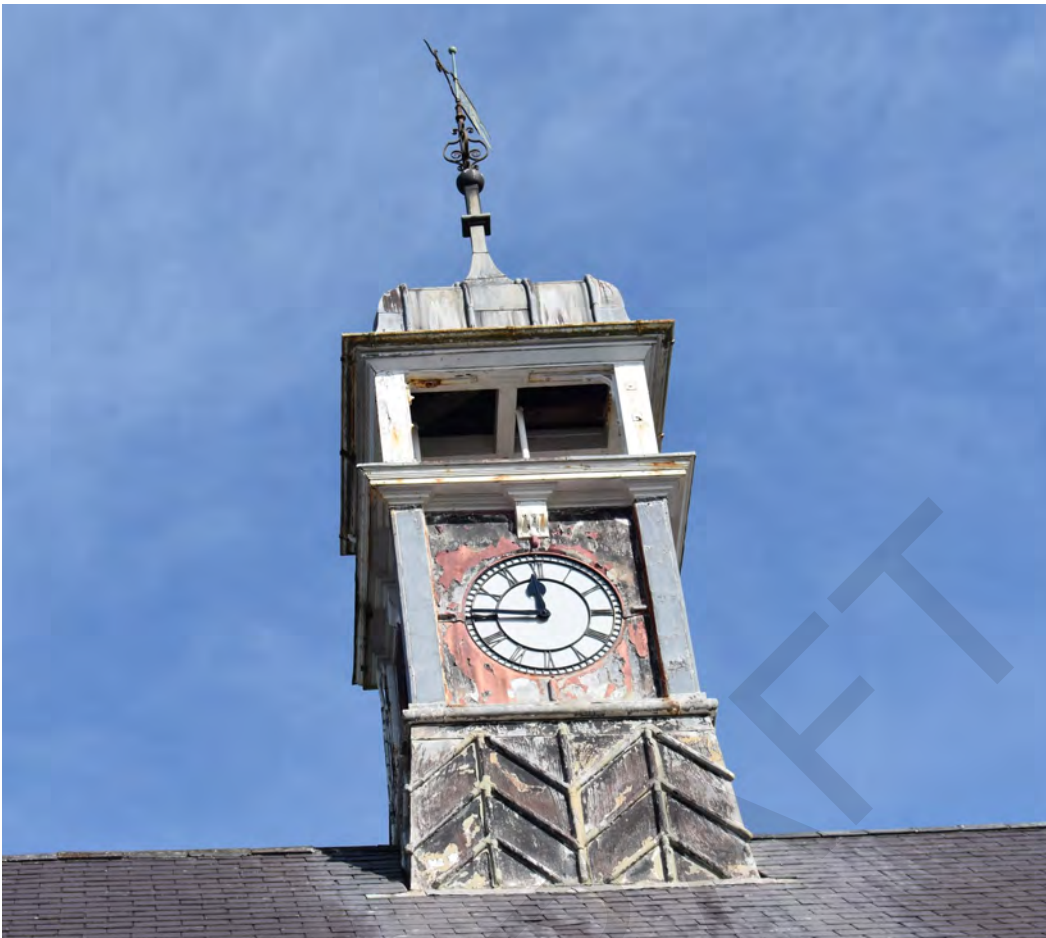
Fig. 16 The Town Hall clock tower is a key architectural feature but is unfortunately in need of some repair
