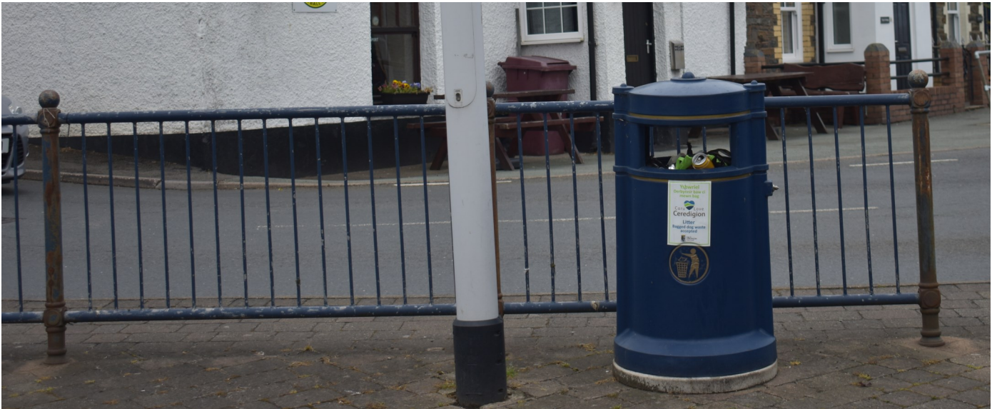
Fig. 27 Appropriately designed safety railings, although in need of some maintenance
