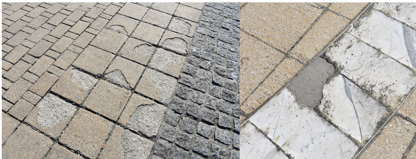
Figs. 12 and 13 Areas of relatively newly resurfaced promenade are starting to fail, in places inappropriate repairs have been undertaken
