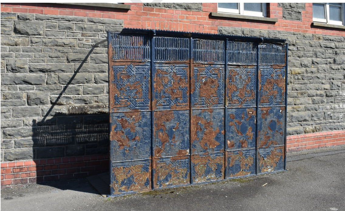
Fig. 6 Unlisted structures with historic interest such as this Victorian urinal could be considered for inclusion on a 'local list'
