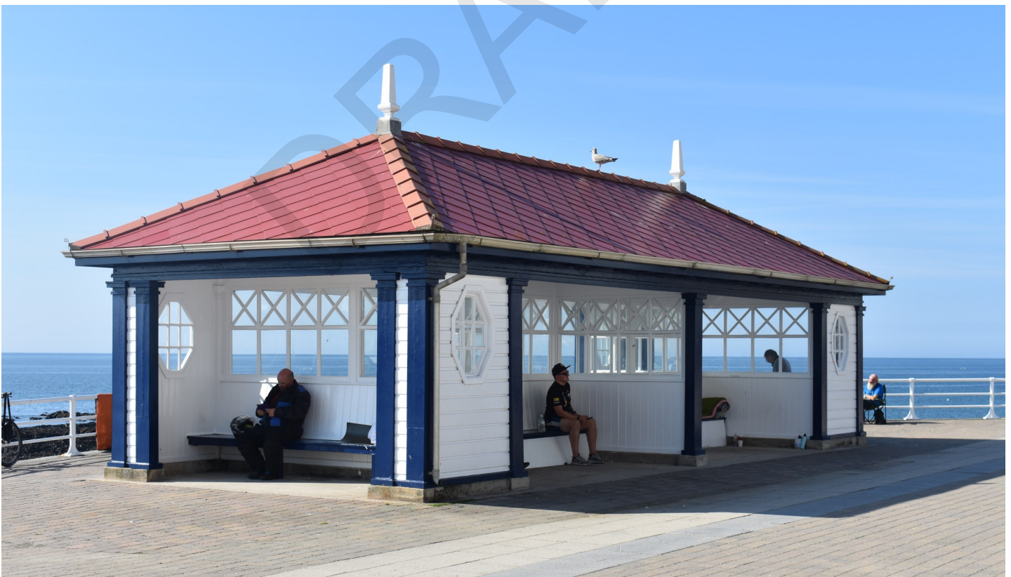
Fig. 7 The 1924 Grade II Listed Bathrock shelter has been subject to several regeneration projects following damage from fierce storms
